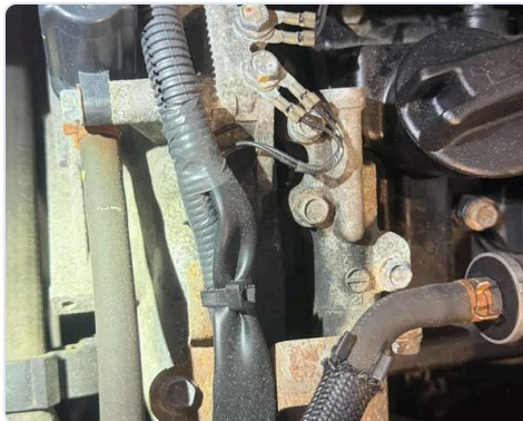
Wiring and grounds
