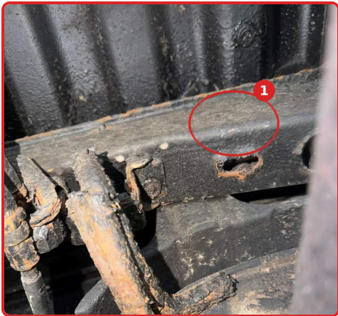
#1 Frame rail rusted through with jagged, scaled hole edges
