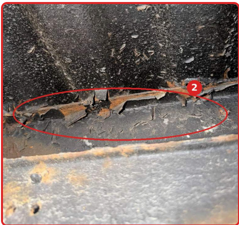
#2 Underbody seam: rust lifting the undercoating
